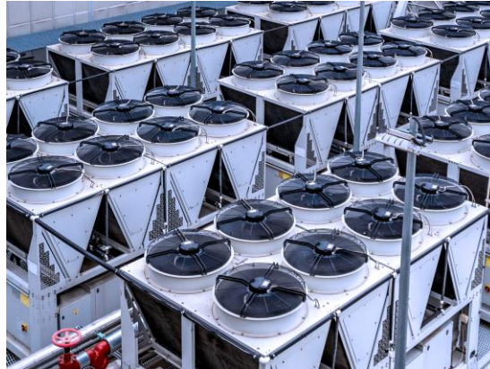
Rooftop chiller plant
